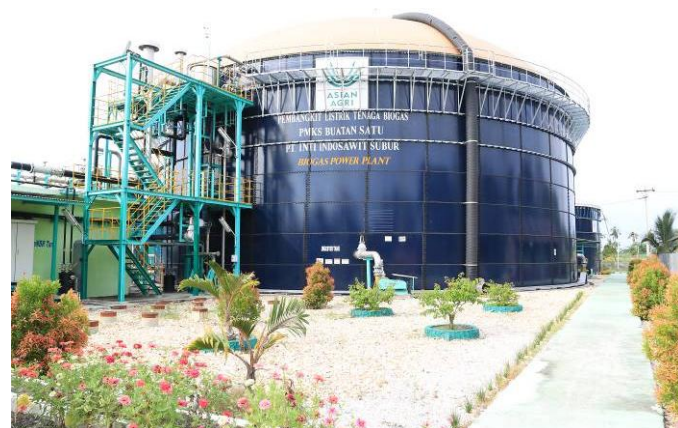
Picture : Methane capture plant.
