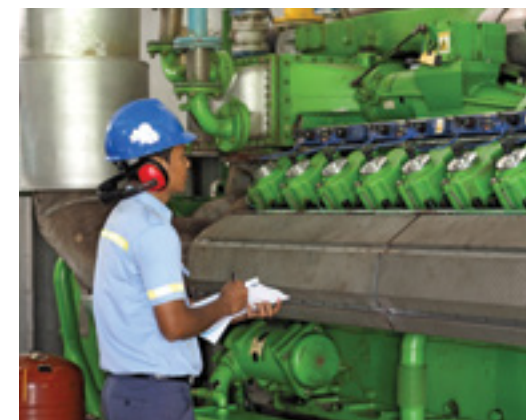
Employee at PT Inti Indosawit Subur biogas power plant in Buatun, Riau
