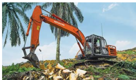
Zero burning method in replanting of oil palm at Buatun Estate, Asian Agri
