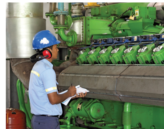
Employee at PT Inti Indosawit Subur biogas power plant in Buatun, Riau
